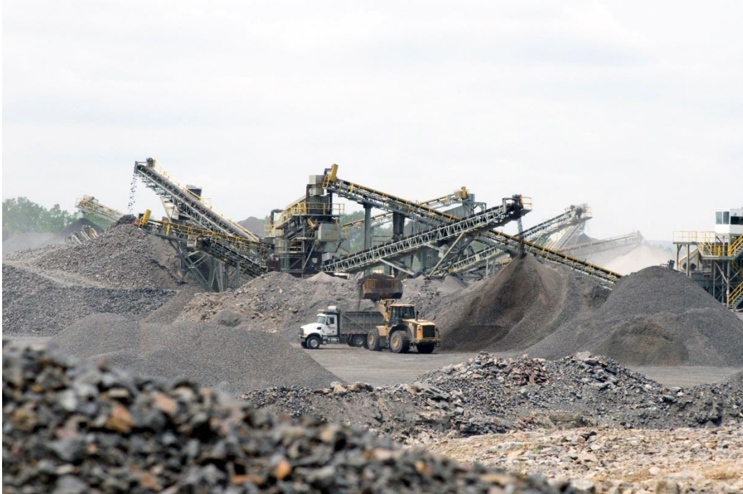
Aggregate processing activity at The H&K Group’s Pottsville Materials facility located in Pottsville, PA.
